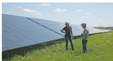
Invenergy's Grand Ridge Energy Center located in LaSalle County, Illinois.
